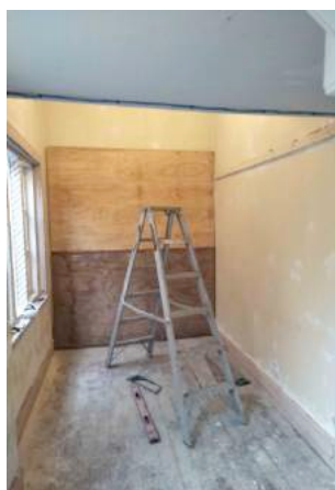
The maintenance room Waiting for stage 2
